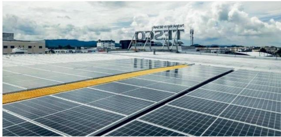
A rooftop view of partially installed solar PV panels on Tesco Jitra, one of the 15 Tesco stores that will soon begin generating clean solar energy. – TESCO
